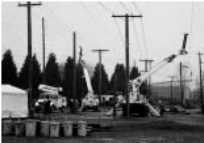
The Robotic Arm allows for safe and efficient repair and replacement of any transmission or distribution system.
