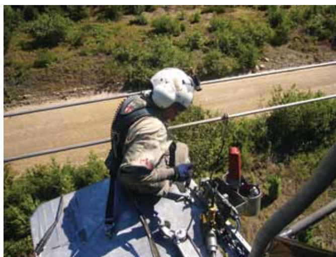
Lineman Don McLellan is shown here working on spacer replacements on the 3L2, 3L5 transmission circuit, Seton Portage - Rosedale substation.
