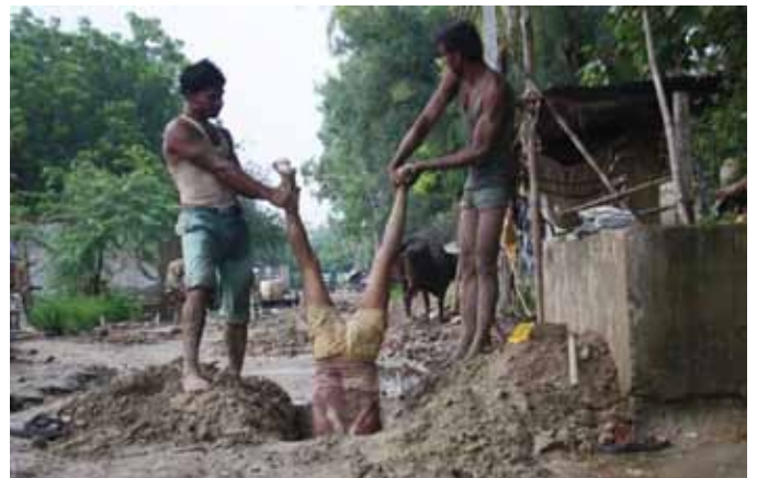
Labourers hold their colleague to install underground electric cables on a roadside at Noida in the northern Indian state of Uttar Pradesh August 27, 2010.
