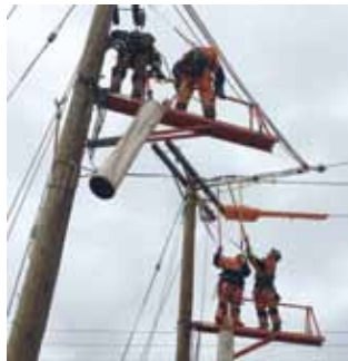
BCH Level 2 Apprentices left to right: Steve Covington & Josh Graham, Ryan Swann & Iain Roby, performing a transfer of a 3 phase DE from one pole to the other using hot stick methods. Photos by Brother Brian Gueldenstern.
