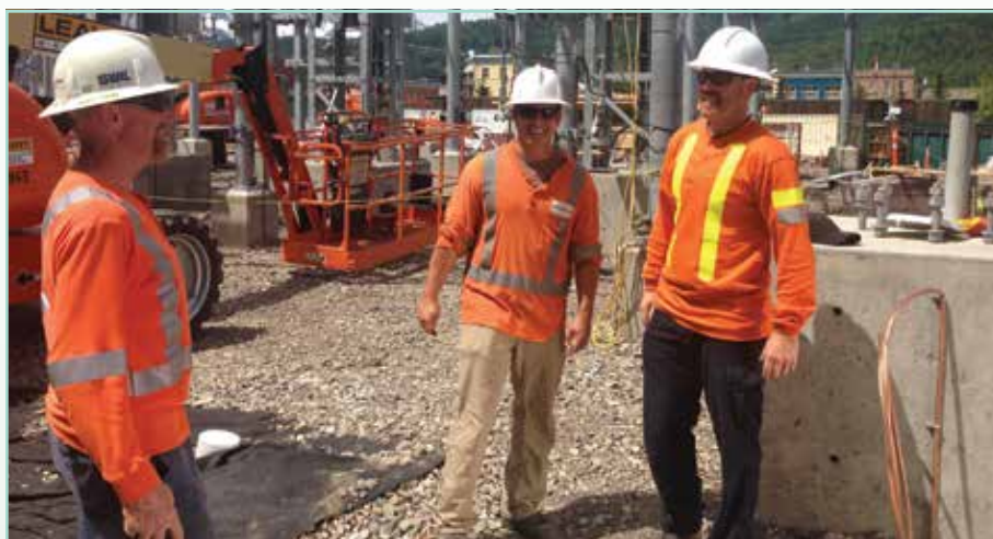
Local 258 members working at BC Hydro's Construction Services Southern Interior crew discussed placement of a new pole for temporary power last June. In the background is the new 25 kV portion of the Fernie substation upgrade project and historic downtown Fernie. From left to right are Brother Dave Hurl, PLT Foreman; Brother Murray Anderson, Civil Sub-Foreman; and Brother Quinn Salt, Electrical Foreman. Thanks to Charlie Kopola, Field Manager, Construction Services, Vernon, for sending the photo to Local 258's Dispatcher Jim McKay who forwarded it to the Hotline.
