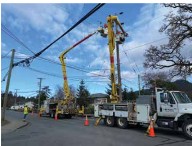
Traffic control providing safety services protecting a BC Hydro crew working at the roadside in Duncan, BC.
