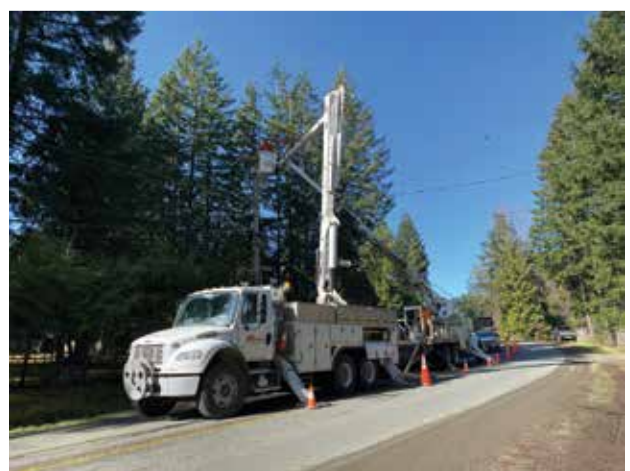
Traffic control providing safety services protecting an Allteck crew working at the roadside in Nanaimo, BC.
